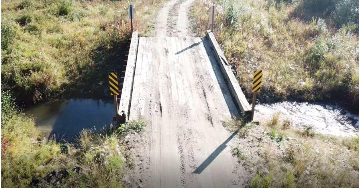
Figure 2.—September 2021 collection of additional field data. Aerial drone imagery of the existing Cache Creek Bridge crossing.
