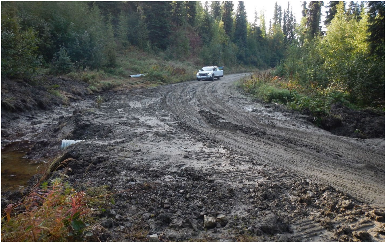
Figure 3.—September 2021 collection of additional field data. Picture of existing roadway conditions observed at Cache Creek Road.
