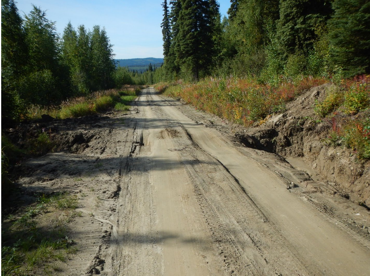
Figure 4.–September 2021 collection of additional field data. Picture of existing roadway conditions observed at Cache Creek Road.
