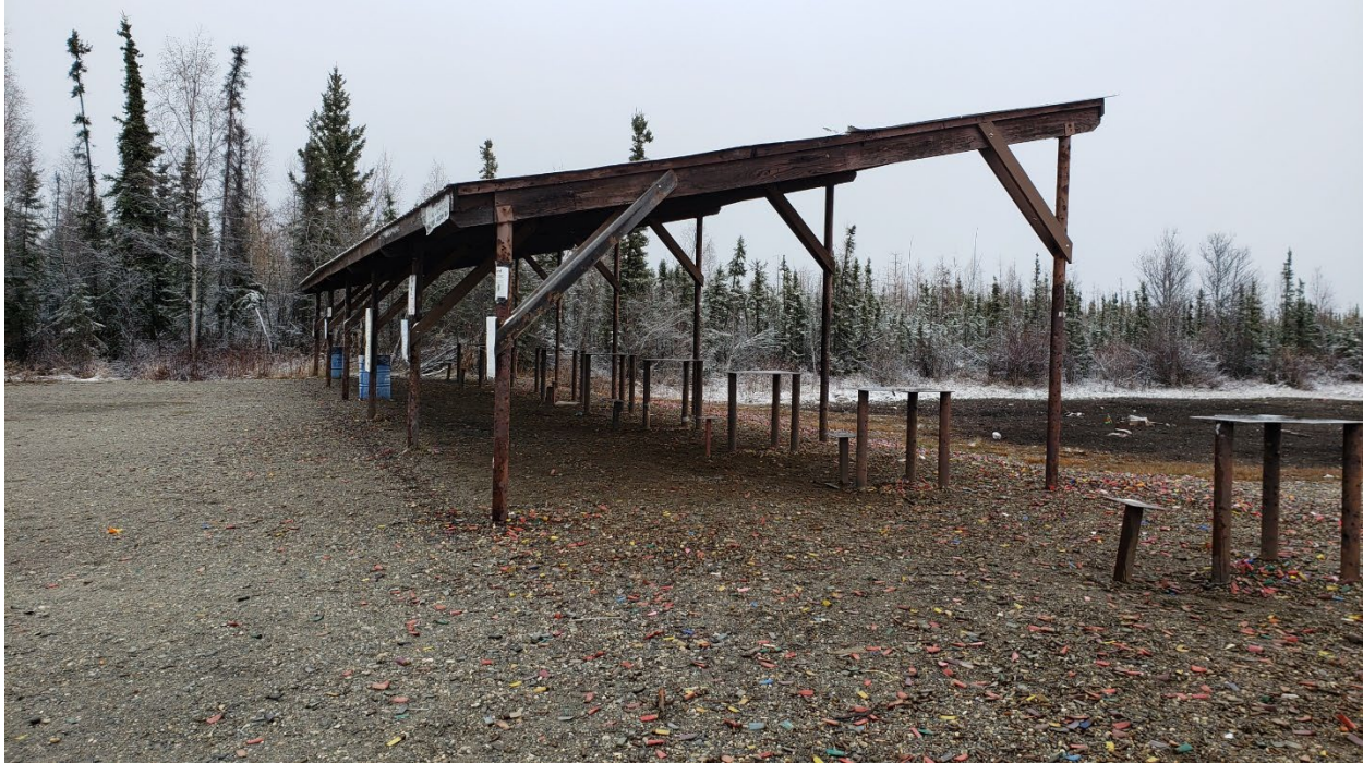
Figure 2.—Existing conditions of the 30+ year old covered roof structure at the 300 yard rifle range.
