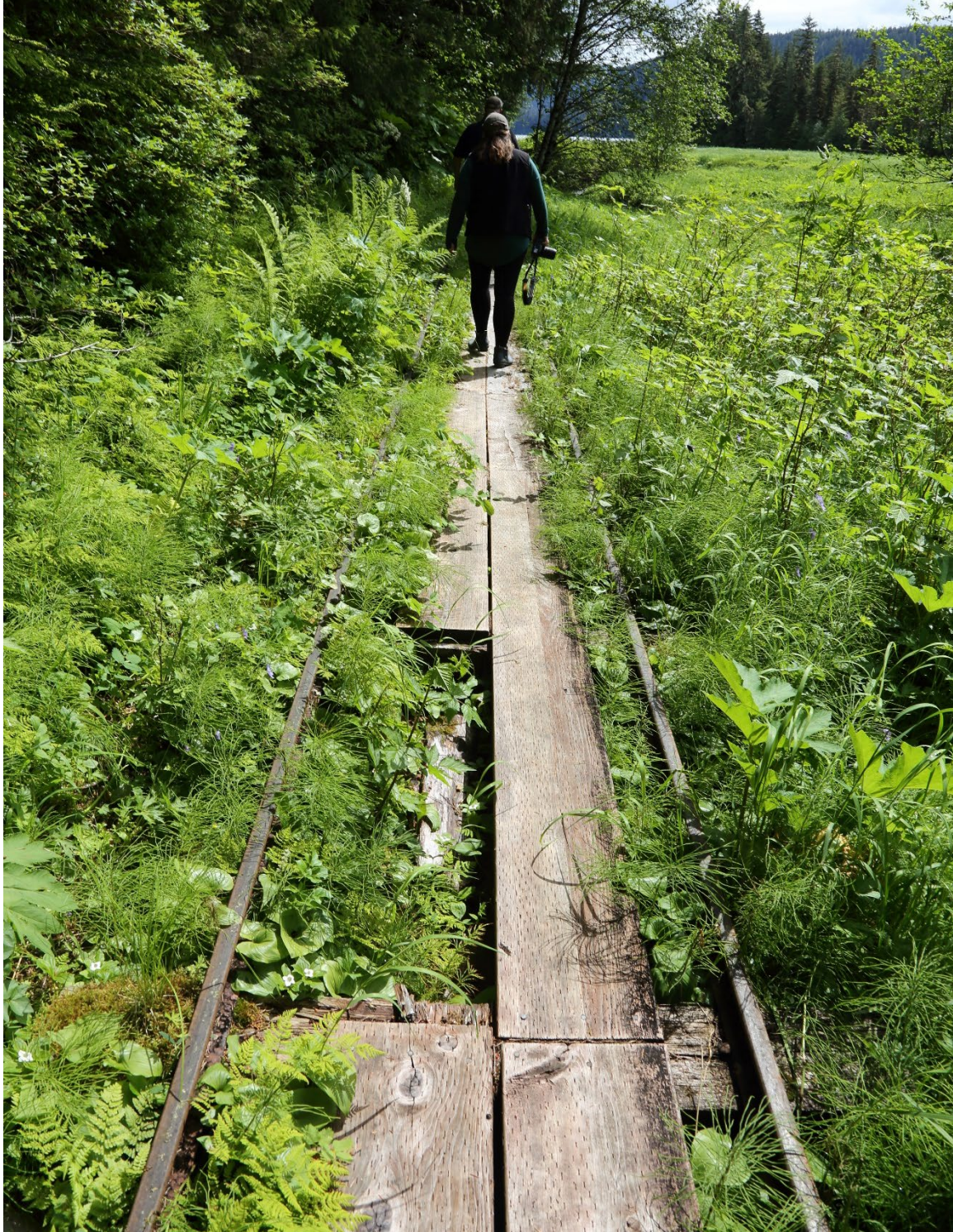
Figure 3.—Existing Oliver Inlet tram conditions.
