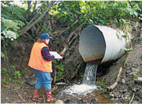
Culverts are inspected to ensure that natural flow and streambed conditions are met to allow safe passage for both adult and juvenile fish. Improperly installed culverts like the one above should be replaced to ensure salmon survival.
