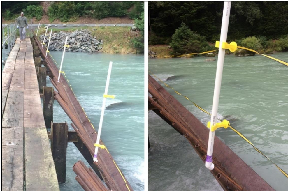
Figure 6.—An electric fence is installed on the front face of the Chilkoot River weir to discourage bears from climbing up on the walkway; the fence is strung between PVC pipes affixed to the top of iron pickets spaced at 3 m intervals. (© 2019 ADF&G.)
