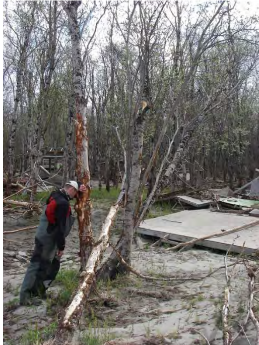
Camp site early season 2009. In this year a large flood during ice out destroyed camp requiring a substantial rebuild. This level of preseason construction is not common, but each year some repairs are required and will test our carpentry skills.
