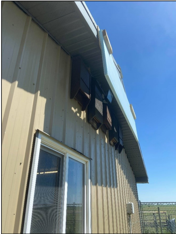
Figure 18. Landowner-installed sunshade -- insulated foam board attached to roof flashing as a temporary sunshade to protect bats during an extreme heat event. Photo by J. Thomson.
